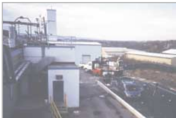
Construction of a Hydraulic Fracture Enhanced SVE System at an Operating Pesticide Plant
