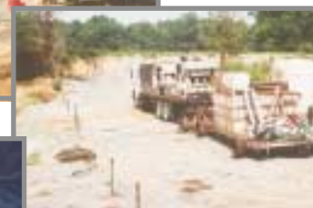
Frac Wells ready for Injection of Iron Slurry Mixture for Reactive Barrier
