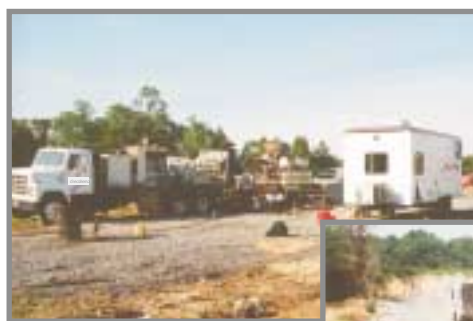
Mixing and Pumping Equipment
