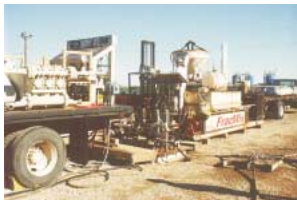
Mixing and Pumping Equipment
